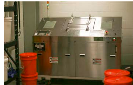
Biodigester for organic waste.
